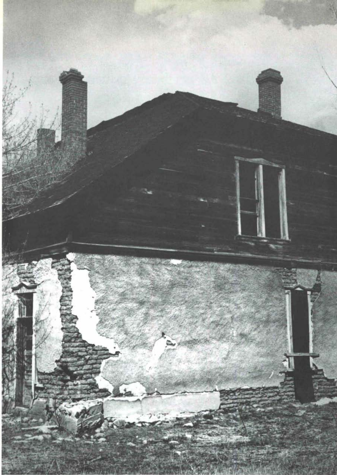
Wooden second story sits on adobe walls. The concrete added at a later date to deter erosion.
